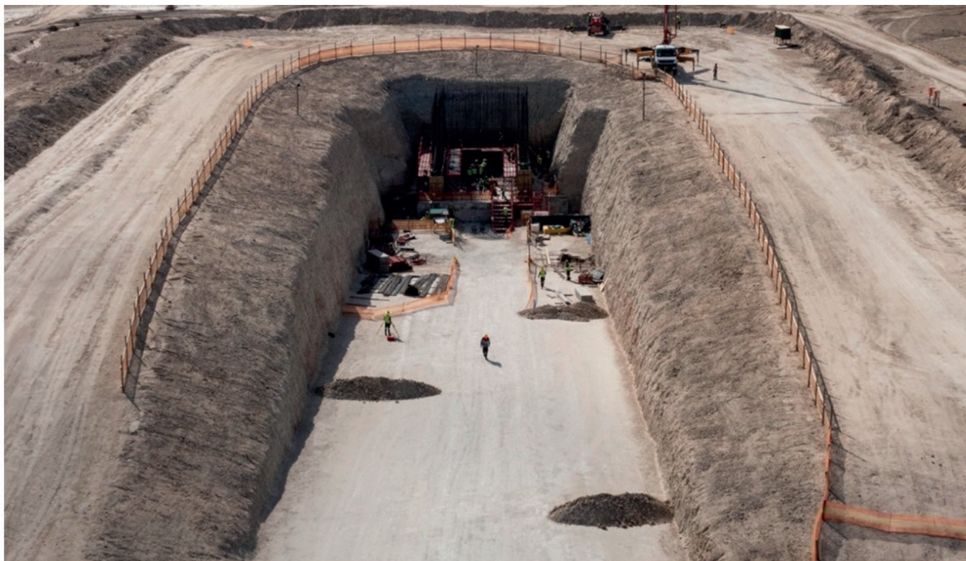
Figure 2: The first concrete pour at the primary crusher site has been completed. A total of 500m 3 was poured at an average flow rate of 40m 3 per hour.
